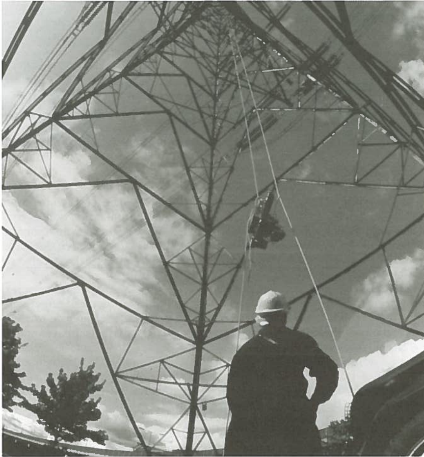
Pylon supporting electric power lines is prepared for a new job: carrying fiber-optic cable. By 2025, there will be a broadband, fiber-optic-based network of networks circling the world. (Assumption 23)
