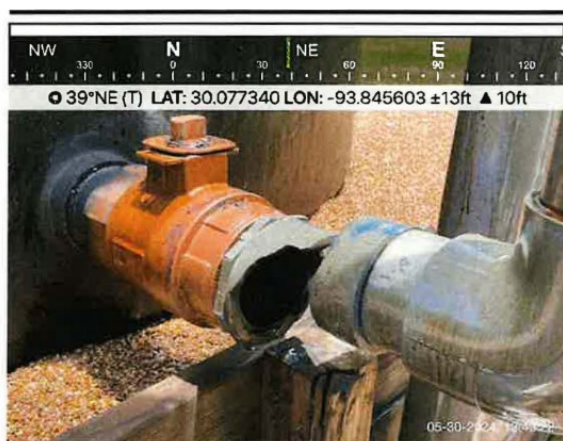
Pic # 5 of broken water leg on gun barrel.
