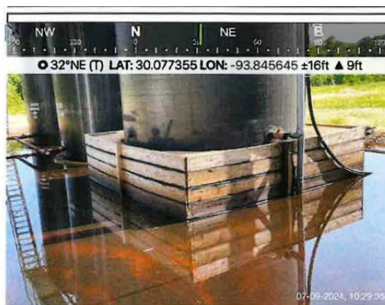
Pic # 1 of oil in fierwall appx 1-1/2" deep Firewall dimension 70 feet x 50 feet. Firewall berm 2-1/2feet with a 5 foot base depyh of fluid in firewall is 2-1/2 inches.
