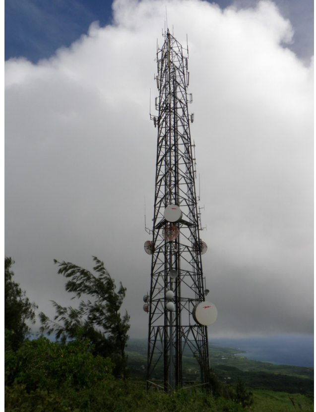
Figure 2-3. Example of a typical communication site on Mt. Tapochau.
